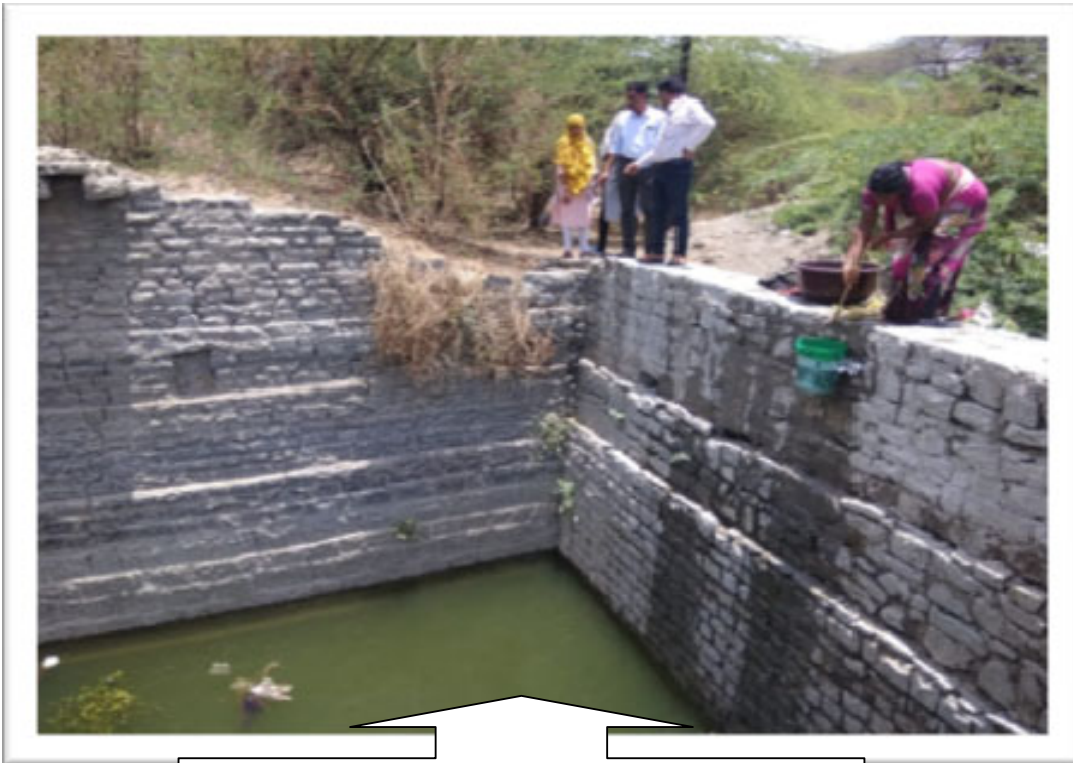
A step well located at Company Bag Required to repair & Desilt
