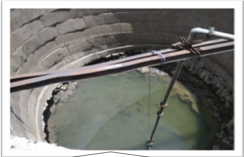
A well located at Company Bag Required to Desilt
