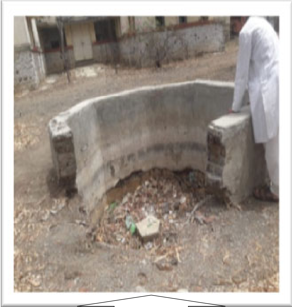
A Well filled by wastages and garbages at pension pura
