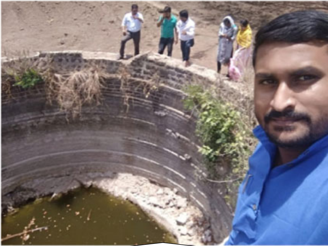
A well located at Company Bag Required to Desilt
