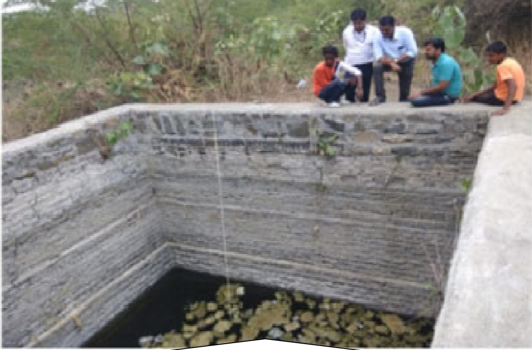
A step well located at Company Bag Required to Desilt
